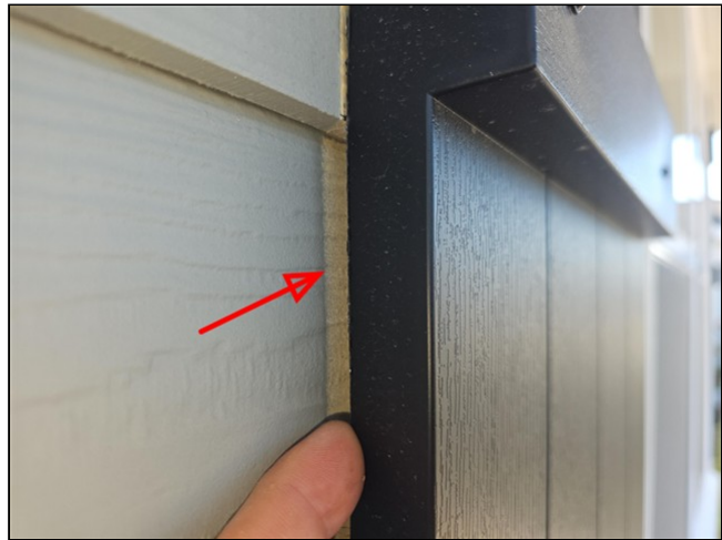
unpainted wall behind decorative shutters on front porch
