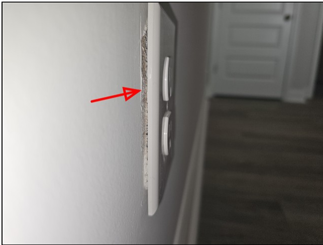
gap between wall and cover plate at multiple interior receptacles and switches
