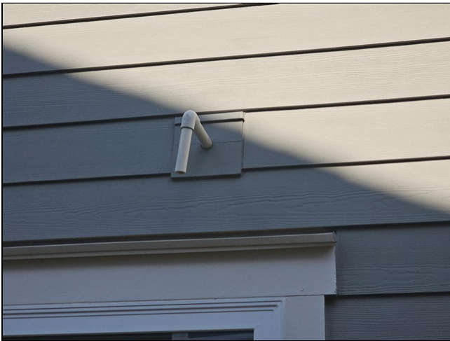
condensation drain line positioned above window on right exterior wall
