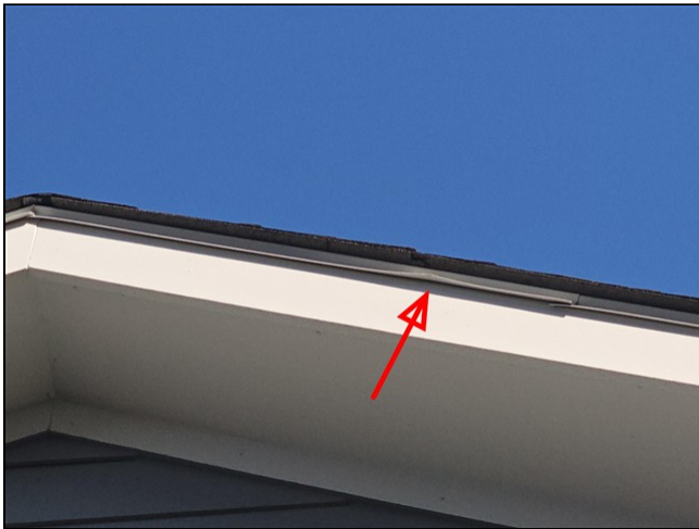
deflected drip-edge flashing at right gable rake
