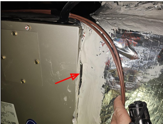
gap in mastic at interior unit allowed air leakage
