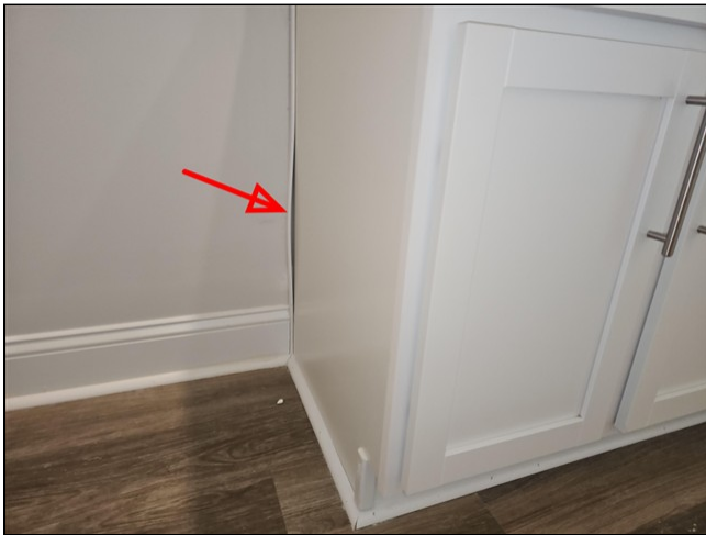
loose cabinet trim in primary bathroom
