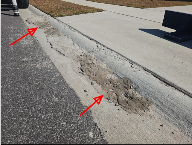
construction debris (hardened concrete) at edge of driveway
