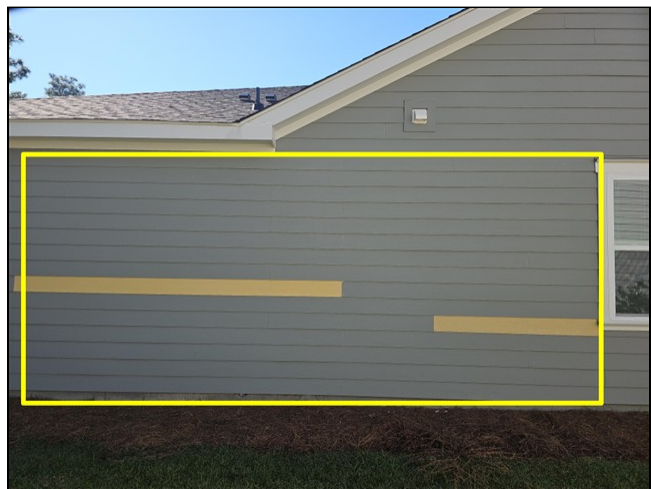
general location of affected siding
