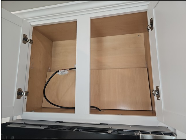
cabinet shelf above microwave not installed
