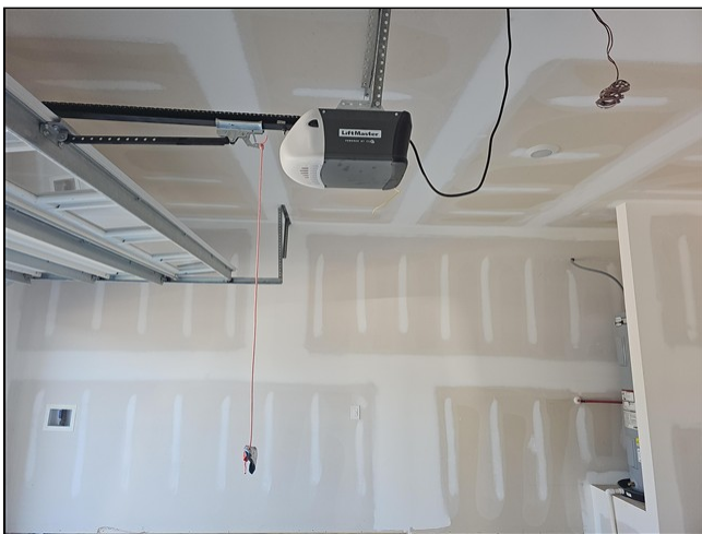
garage door opener was inoperable / may require additional programming
