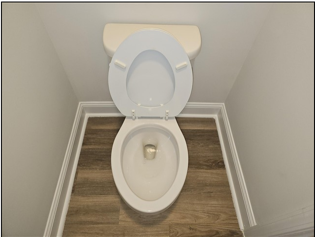
primary bathroom toilet: weak flush
