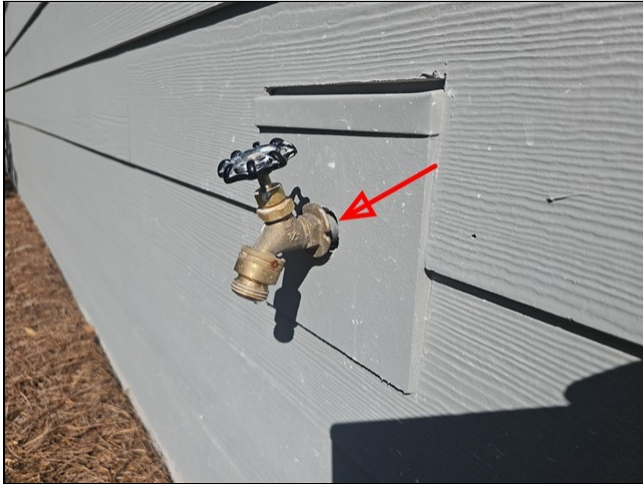
right-rear corner: unsealed hose bib
