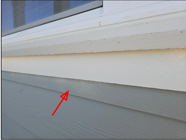
paint over-spray on wall at front porch
