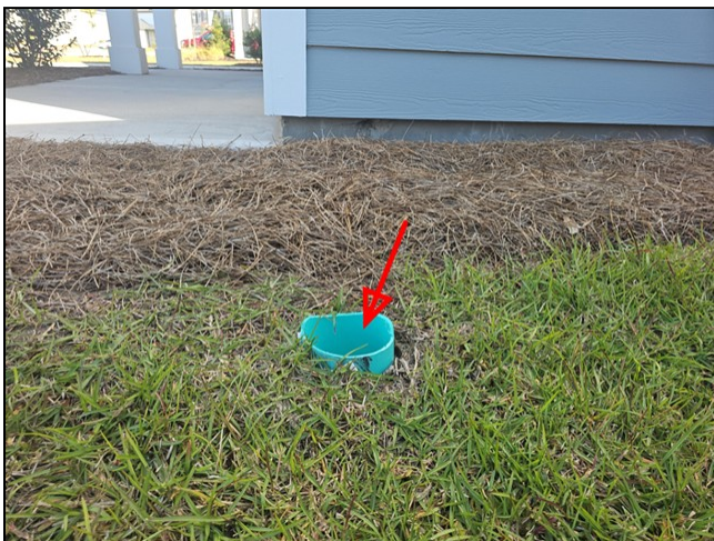
right-front corner: un-capped plumbing drain cleanout
