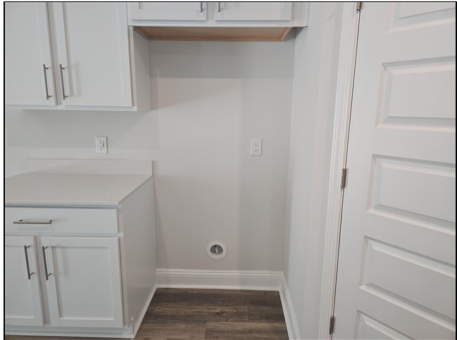
refrigerator not installed
