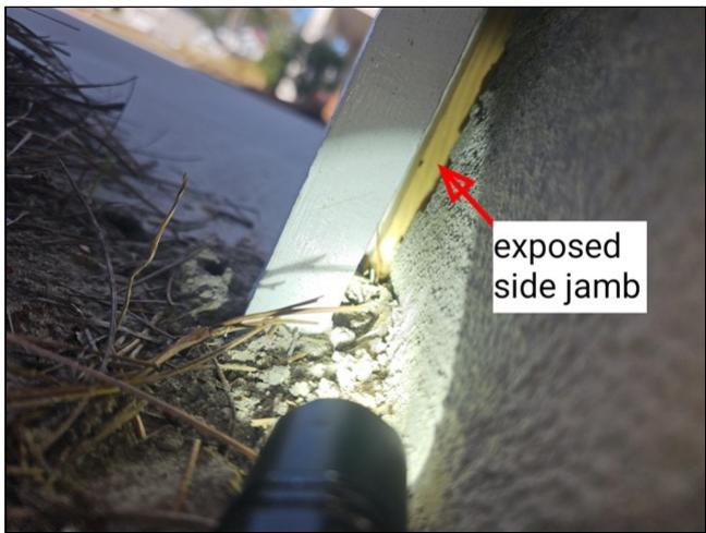
lower exterior corners at garage door were unsealed
