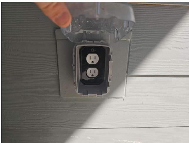
loose receptacle at patio
