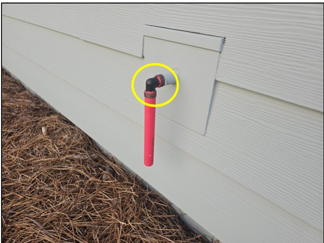
excessive amount of connections in TPR drain line
