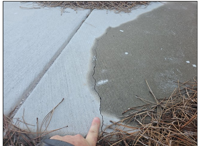
hairline crack in front walkway
