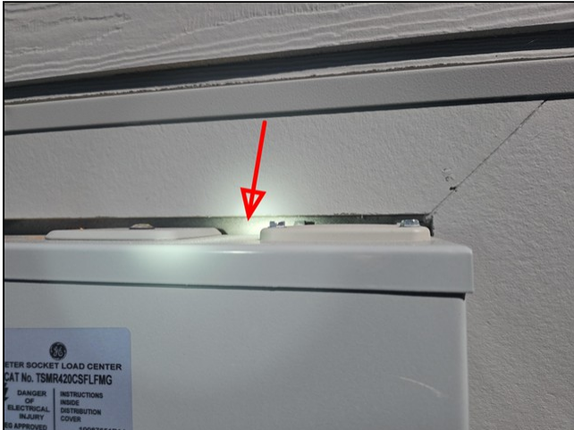
poorly sealed around edges of panel
