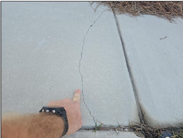
hairline cracking in front walkway
