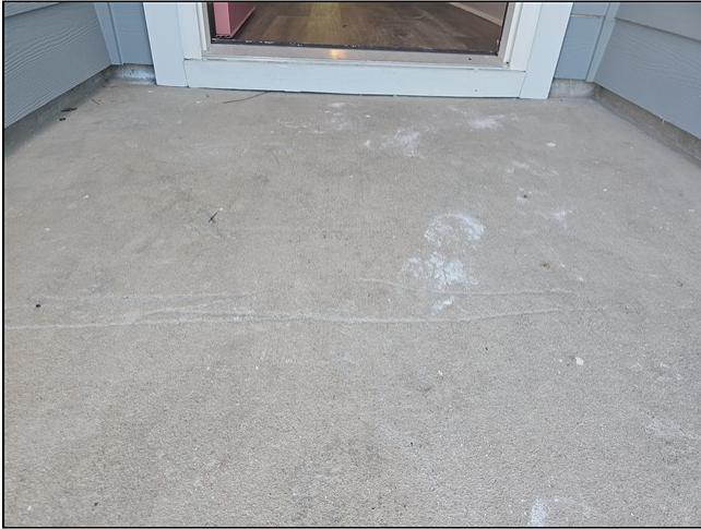
front porch: gouges in concrete
