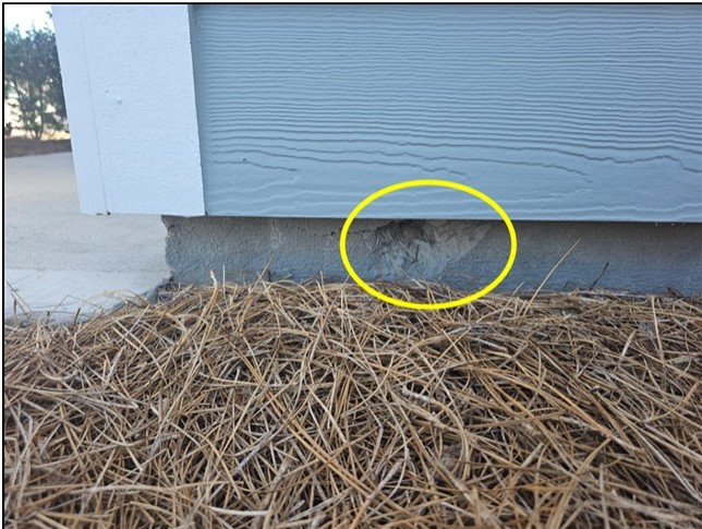
chipped concrete at multiple locations around edge of foundation
