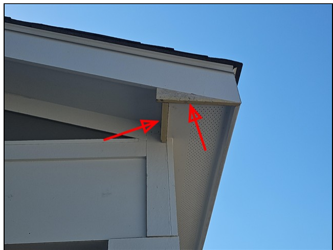
unpainted trim at front porch overhang
