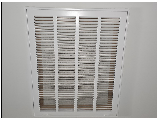
filters were clogged
