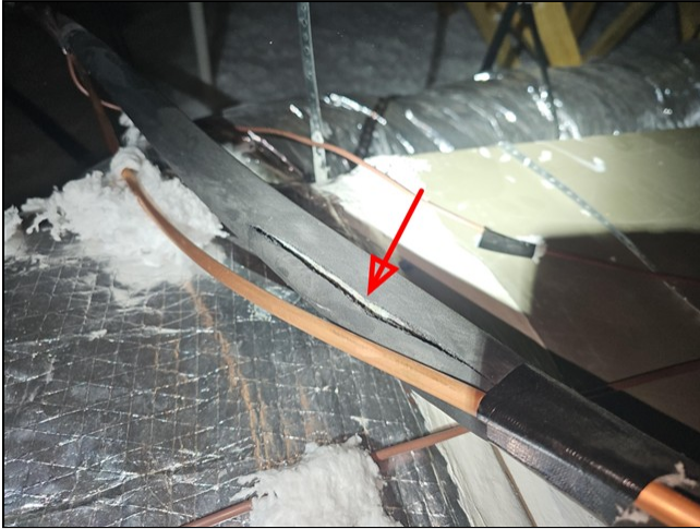
gaps in refrigerant line insulation in attic
