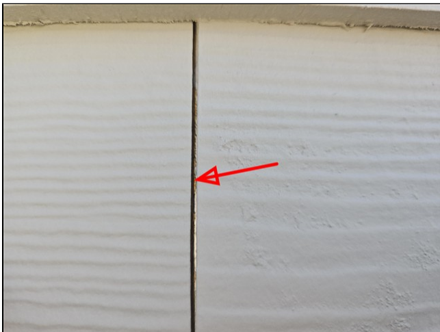
manufacturer-recommended flashing was not visible behind siding butt joints
