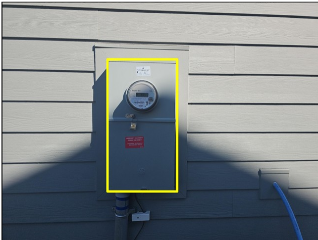
service panel installed directly to wall, recessed within flashed mounting block
