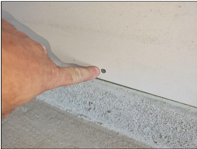
unsealed fasteners in garage drywall that reduce firewall effectiveness
