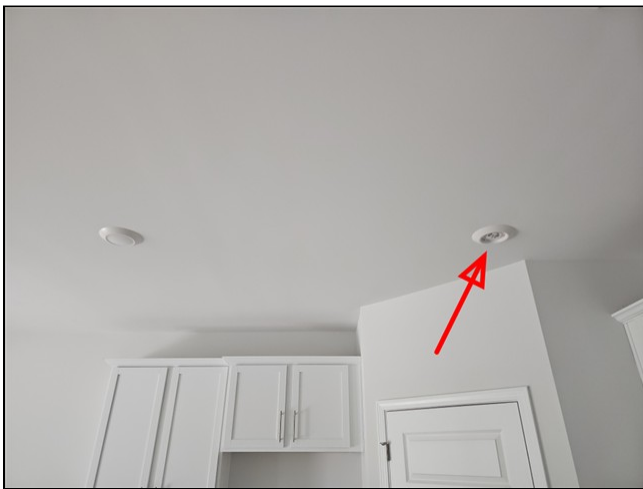
kitchen: recessed light fixture cover was missing
