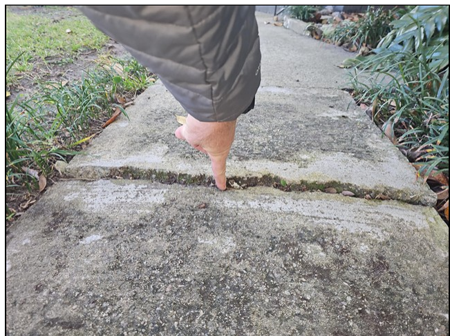
offset crack l'm front walkway
