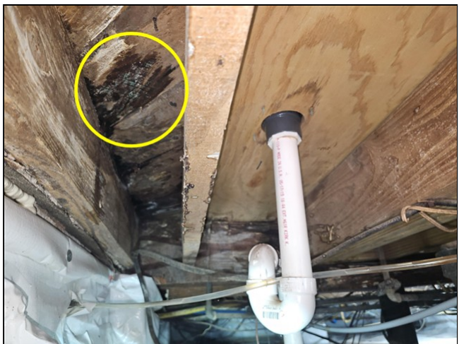
moisture-staining on sub-floor beneath bathroom
