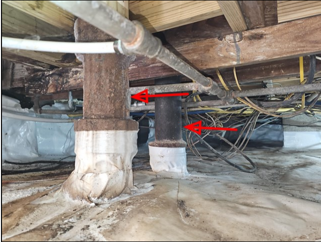
older cast iron drains; recommend sewer scope (standard)
