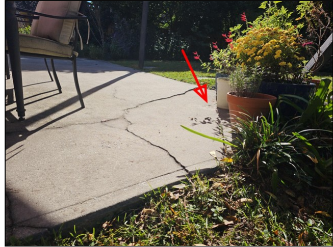
patio: corner of concrete slab cracked & settling
