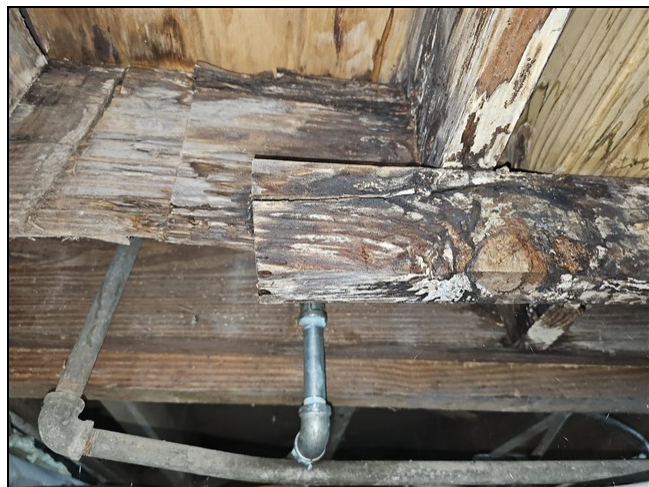
water damage to sub-floor framing due to leak beneath bathroom
