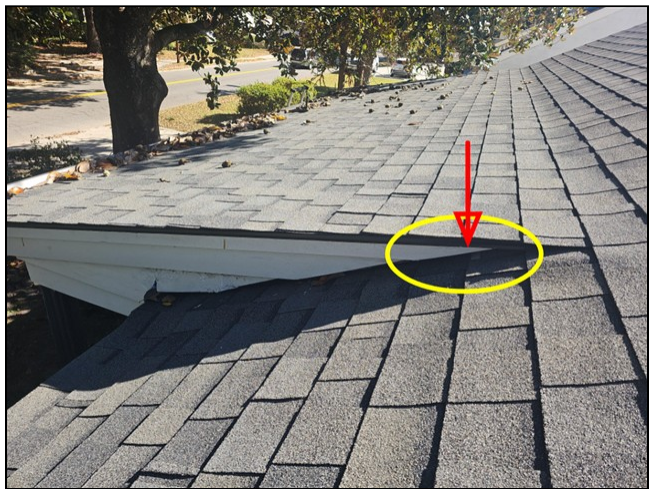
flashing missing where at junction of primary roof and front porch overhang
