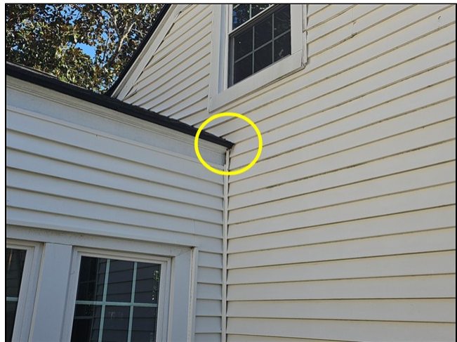
right side: kickout flashing missing
