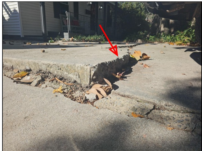
significant cracking in concrete driveway
