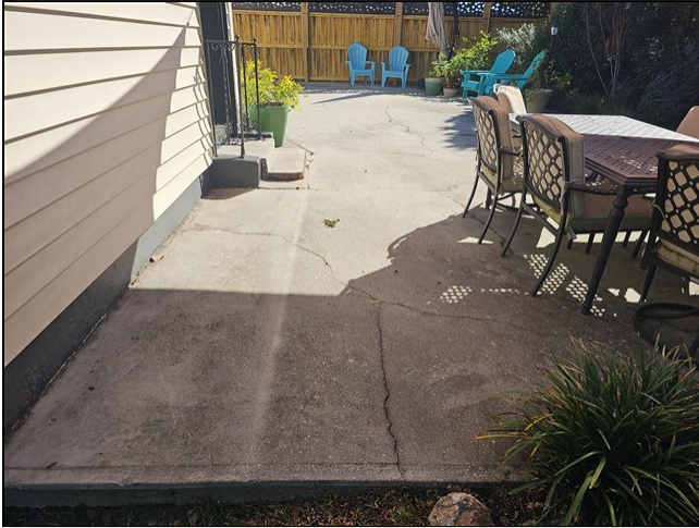
widespread cracking in concrete patio
