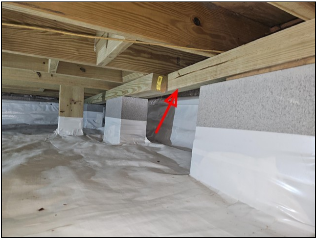
apparent foundation repairs: recommend acquiring documentation from seller
