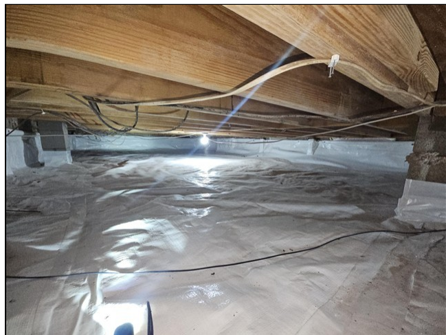
no support piers installed at front-right corner in crawlspace
