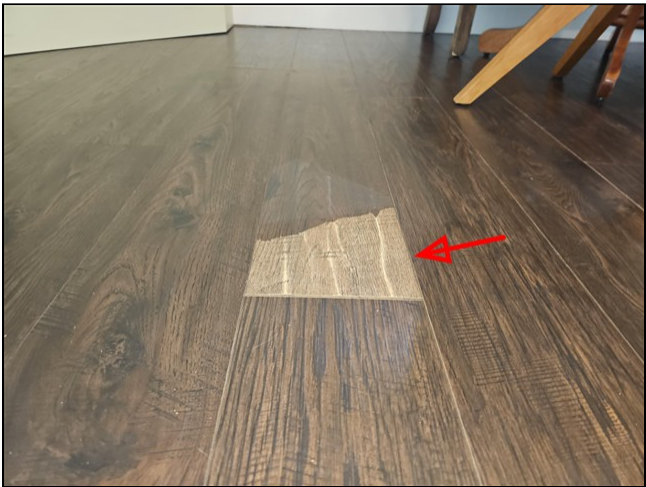
delaminated flooring in kitchen
