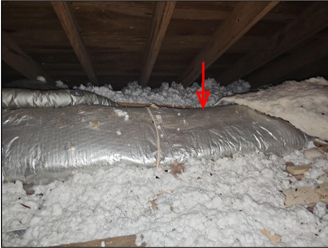
flattened, constricted HVAC duct in bonus room attic
