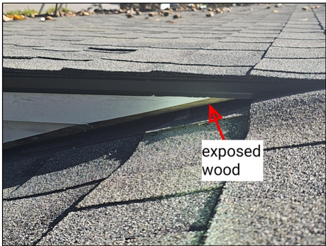
flashing missing where at junction of primary roof and front porch overhang (zoom view)
