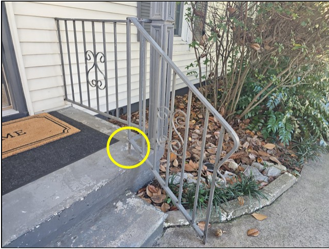
front porch: railing post base was detached, railing was loose
