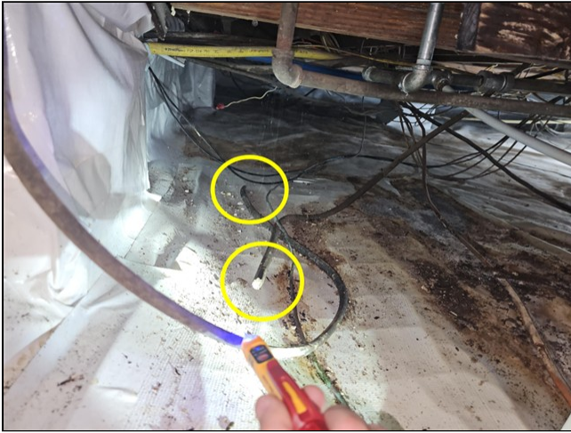
hazardous electrical wiring in crawlspace
