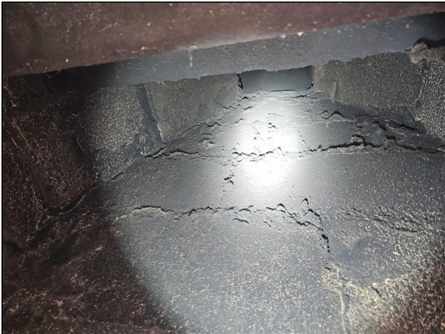
chimney flue had marginal buildup
