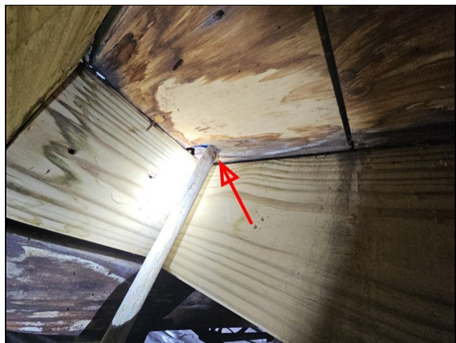
corroded galvanized water supply pipe surrounded by moisture-stained wood
