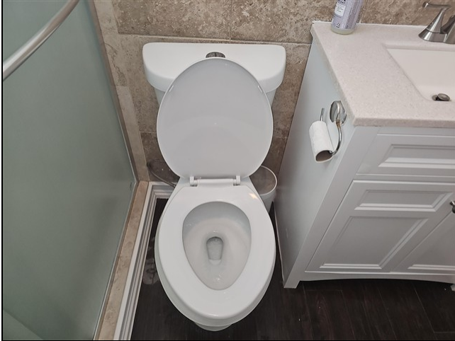
bathroom: loose toilet
