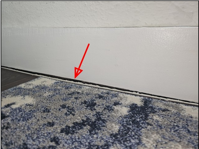
floor-to-wall separation in guest bedroom (left side of home)
