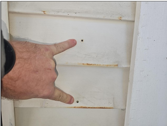
unsealed holes in siding at front porch
