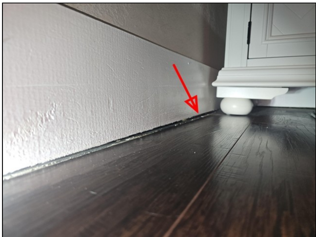
floor-to-wall separation in primary bedroom (left side of home)
