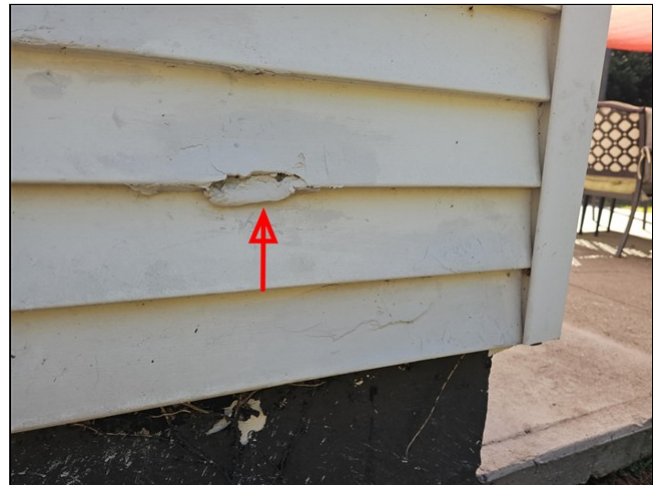
minor siding damage at right-rear corner
