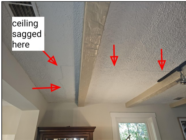
living room ceiling: sagged & cracked
