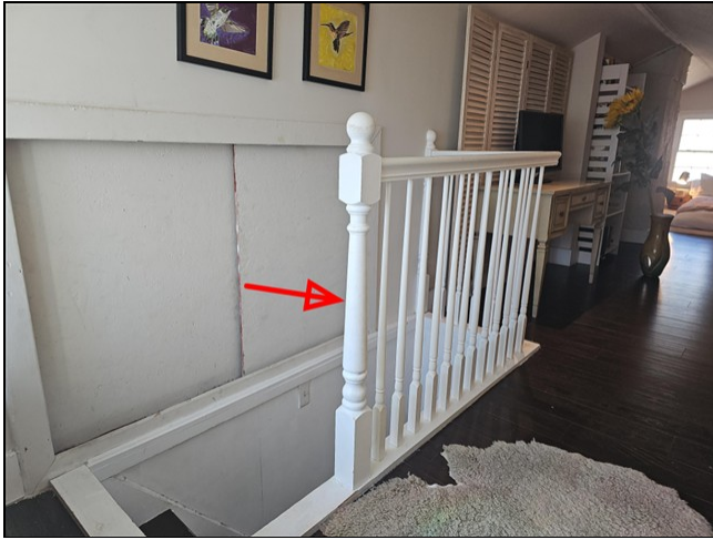
loose newel post at upstairs railing
