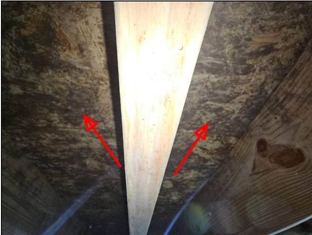
apparent mold growth on OSB sub-floor at the front-right corner area within the crawlspace
