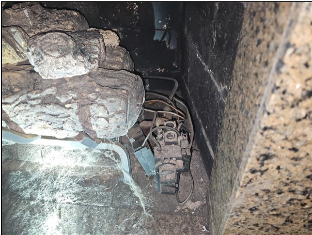
older fireplace controls that appear to have been unused for an extended period
