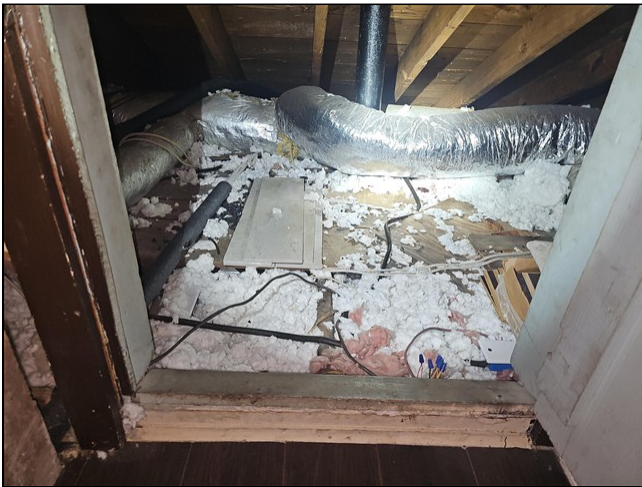
electrical wiring was precariously installed at attic entrance
