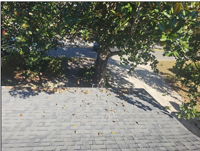
tree debris buildup on front porch overhang
