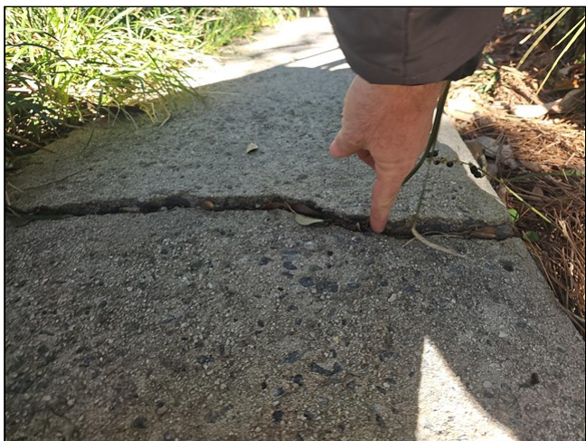
offset crack in front walkway
