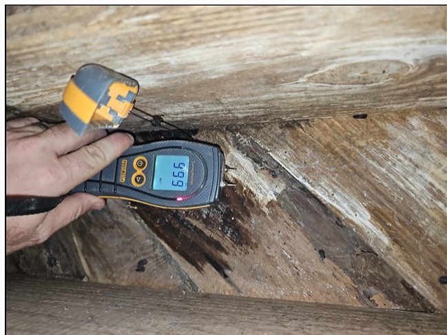
elevated moisture levels on sub-floor at areas where there was moisture staining on wood
